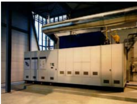
Sistema SOFC Westinghouse 100 kW
